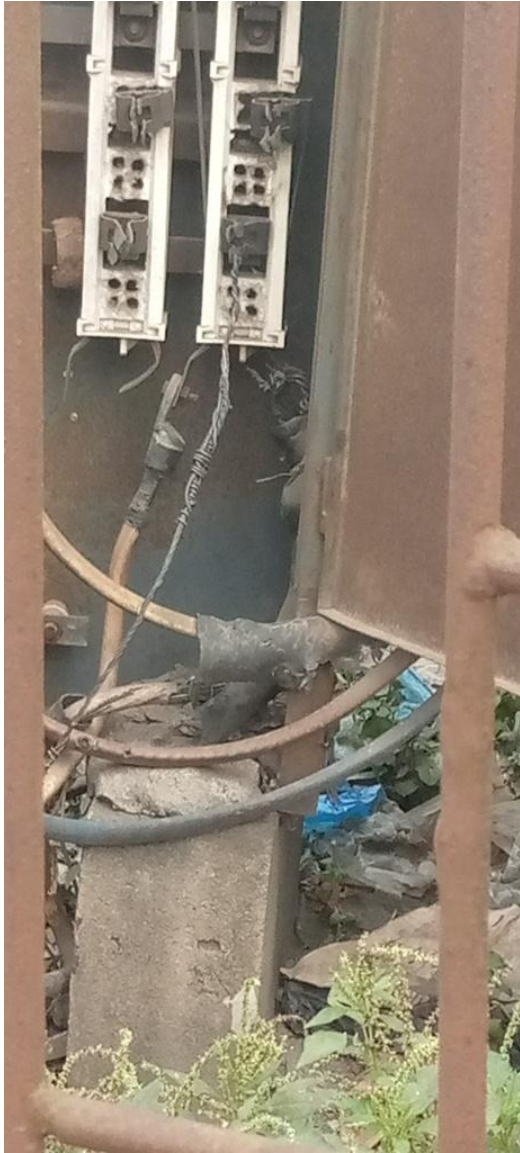
Figure 1: A damaged feeder pillar of a transformer
