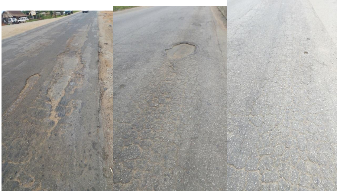
Fig1: Typical Pavement Deformations found in the Study Area
