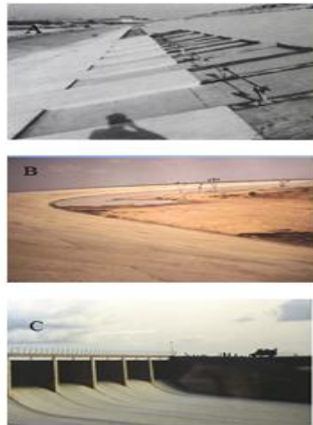
Figure 16: (A): side view geosynthetic liner, (B): upstream view of dam, (C): Dam completion
